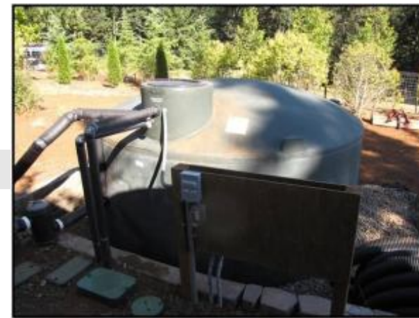
A 5,000-gallon storage tank in the back of the house holds roof runoff to be used for irrigation
